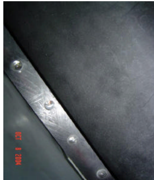
View of LED's mounted inside cove/gill
